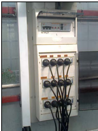
Fig. 2: The main switch of the automated system.
