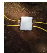
Fig.6 Underground Pressure Sensor
