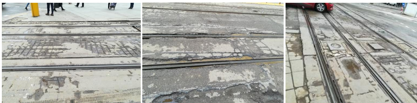
Fig.2 Emergency condition of pavement and concrete panels
