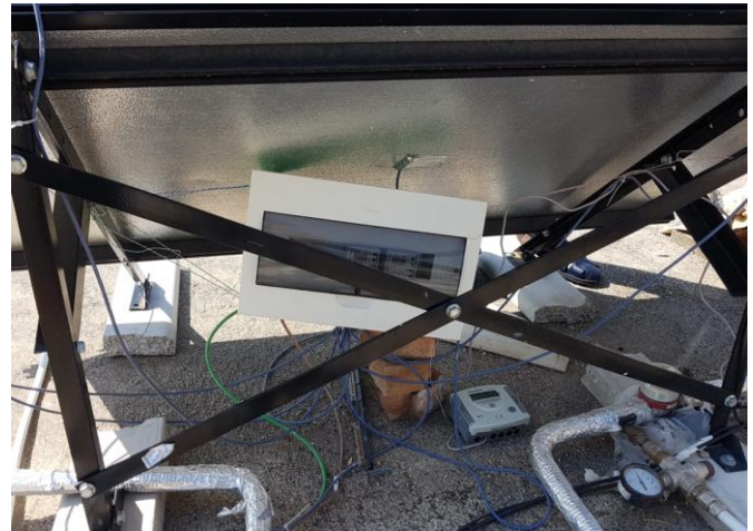
Fig.4 View of the PV/T panel process installation devices
