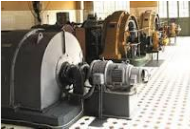
Fig. 2 A general view of the machine room of the HPP 'Enina'.
