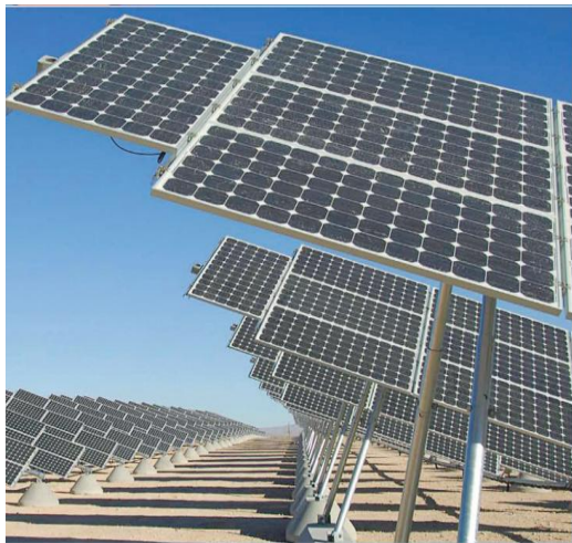
Fig. 9: Nellis Solar Photovoltaic Power Plant with power 14.2 MW (USA) [20, 25]
