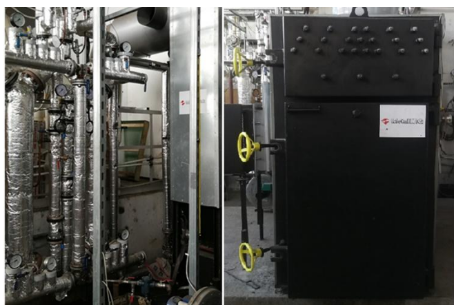
Fig. 1 Tested object - biomass boiler fueled by gray straw..
