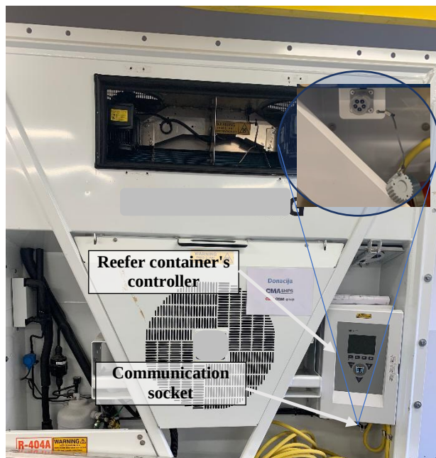
Fig. 10. Reefer container used for communication testing purposes
