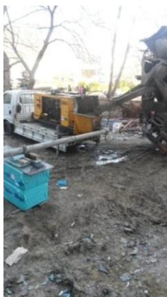
Photo 2 Part of the technological equipment
