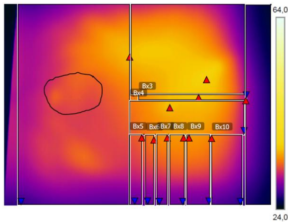
Fig. 15. Presence of a defect (warmer section) on the wall of the beehive.
