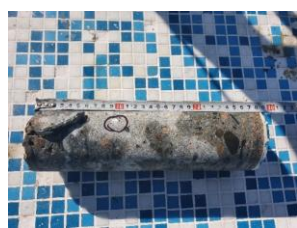
Photo 6 Bottom slab core №3 with length 25 cm (lower steel reinforcement Ø8 cm, located at 17 cm from the upper edge of the bottom, only)
