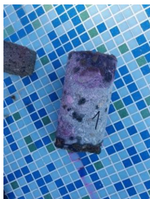
Photo 7 Zero concrete carbonation established by colorization method
