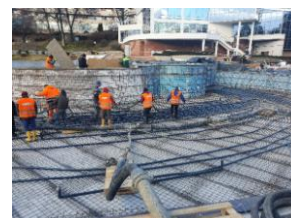
Photo 14 Piping for concrete horizontal transport
