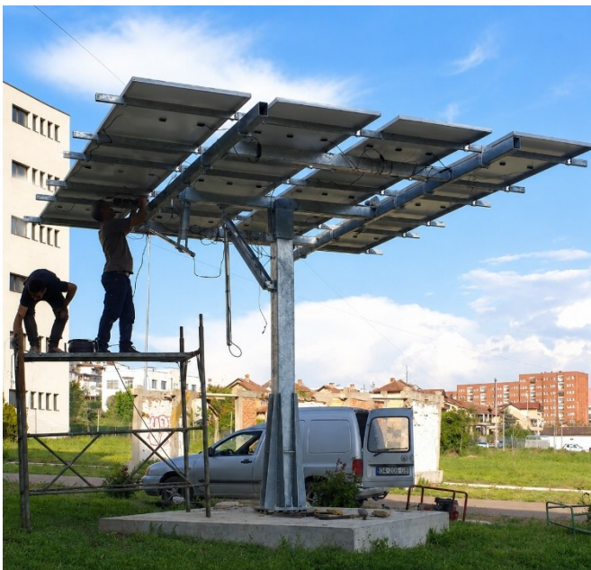
Fig. 17 Final dual-axis solar tracking system
