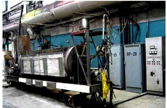
Fig.2 Pilot plant to produce rare-earth elements, molybdenum trioxide, calcium molybdate and to make full utilization of sulfur dioxide
