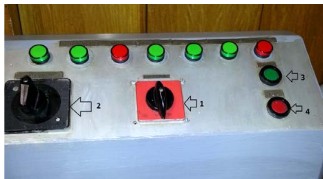
Fig.5 Burner control panel
