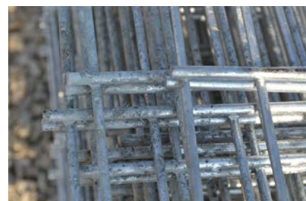
Figure 4 Panels with dross, flux, peeling and spaling
