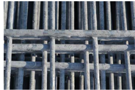
Figure 2 excess materials (zinc coating) on the surface
