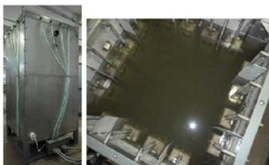
Fig. 19. MO-152 decontamination unit at the Kalinin NPP
