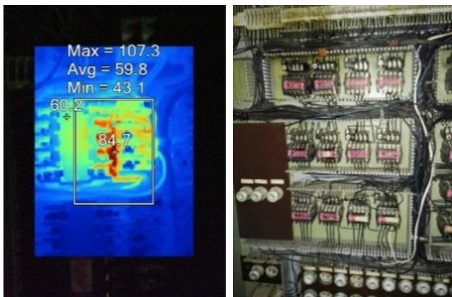
Fig. 3 Thermal image (left) and corresponding visible-light image (right) of the detected exception (poor contacts of worn contactors). [21, 22]
