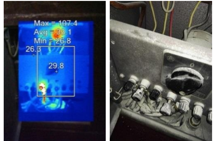
Fig. 1 Thermal image (left) and corresponding visible-light image (right) of the detected exception (hot spot on one of the active phase terminals). [21, 22]
