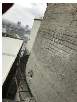
Photo 2 LIGHT SODA SILOS "4" & "5" typical concrete damages
