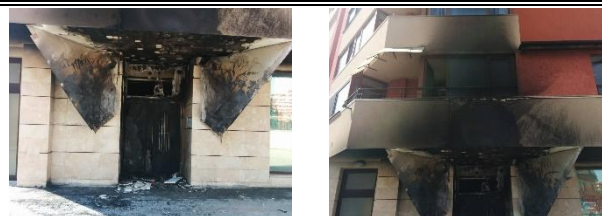
Fig. 1. Fire in a residential building in Sofia, housing estate Mladost 3, covered with thermal insulated panels
