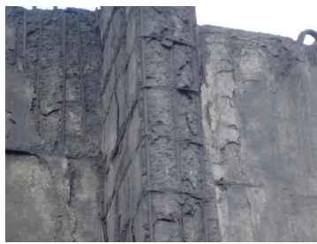
Photo 3 Severe structural damages
