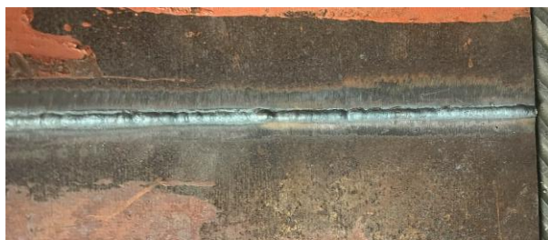
Fig. 11 Detail of the boiled root cutout from pipe No. 2
