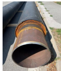
Fig. 2 Pipe sample No. 2 from the new hot water pipe
