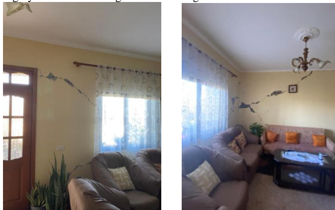
Fig. 5 Building 4 damage around openings.
