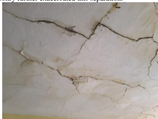
Fig. 6 Building 2 slab degradation and separation from walls.
