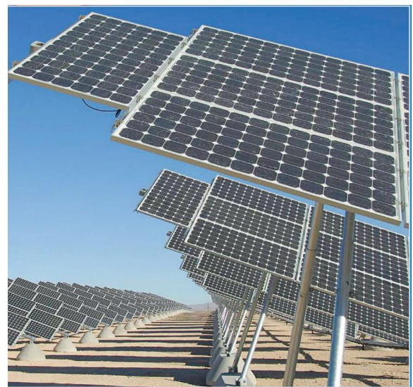
Fig. 3: Nellis Solar Photovoltaic Power Plant with power 14.2 MW (USA) [34,45]
