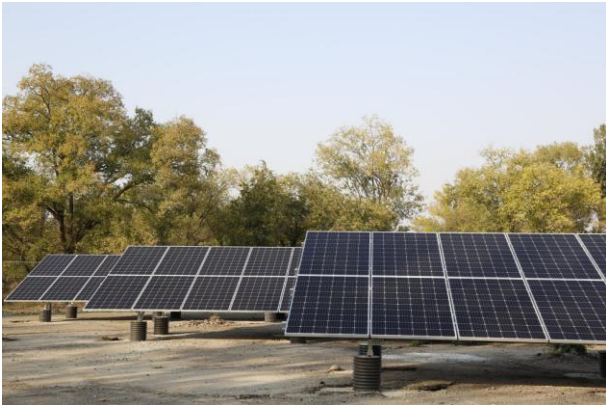
Fig. 9. Solar panels (SP) from 100 kW installed in Krcanisi Park near Tbilisi [10]
