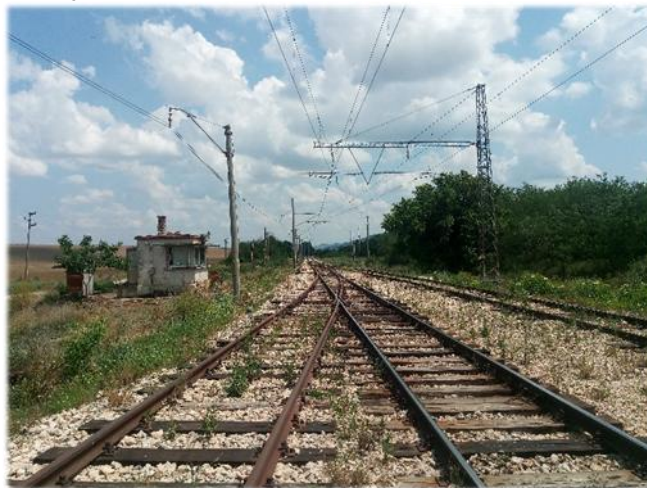
Fig. 9 Catenary line crossing
