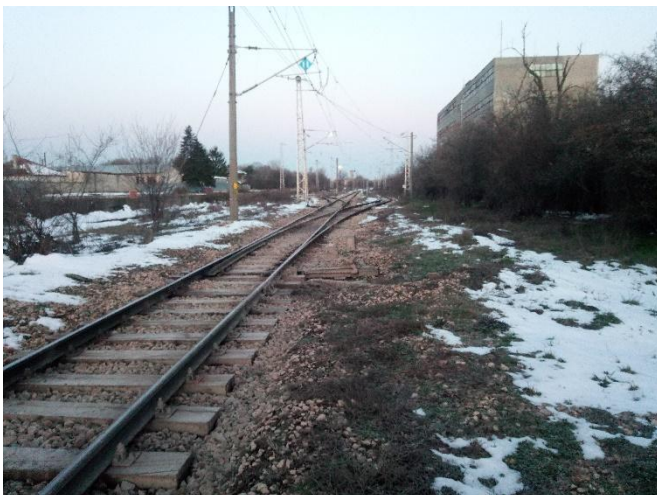
Fig. 5 Switches No. 2 and 4, Razgrad station
